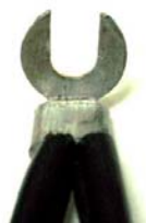
Fig.3: Pigtail tamping damage. Poor tamping causes a "Hot Joint" during operation.
