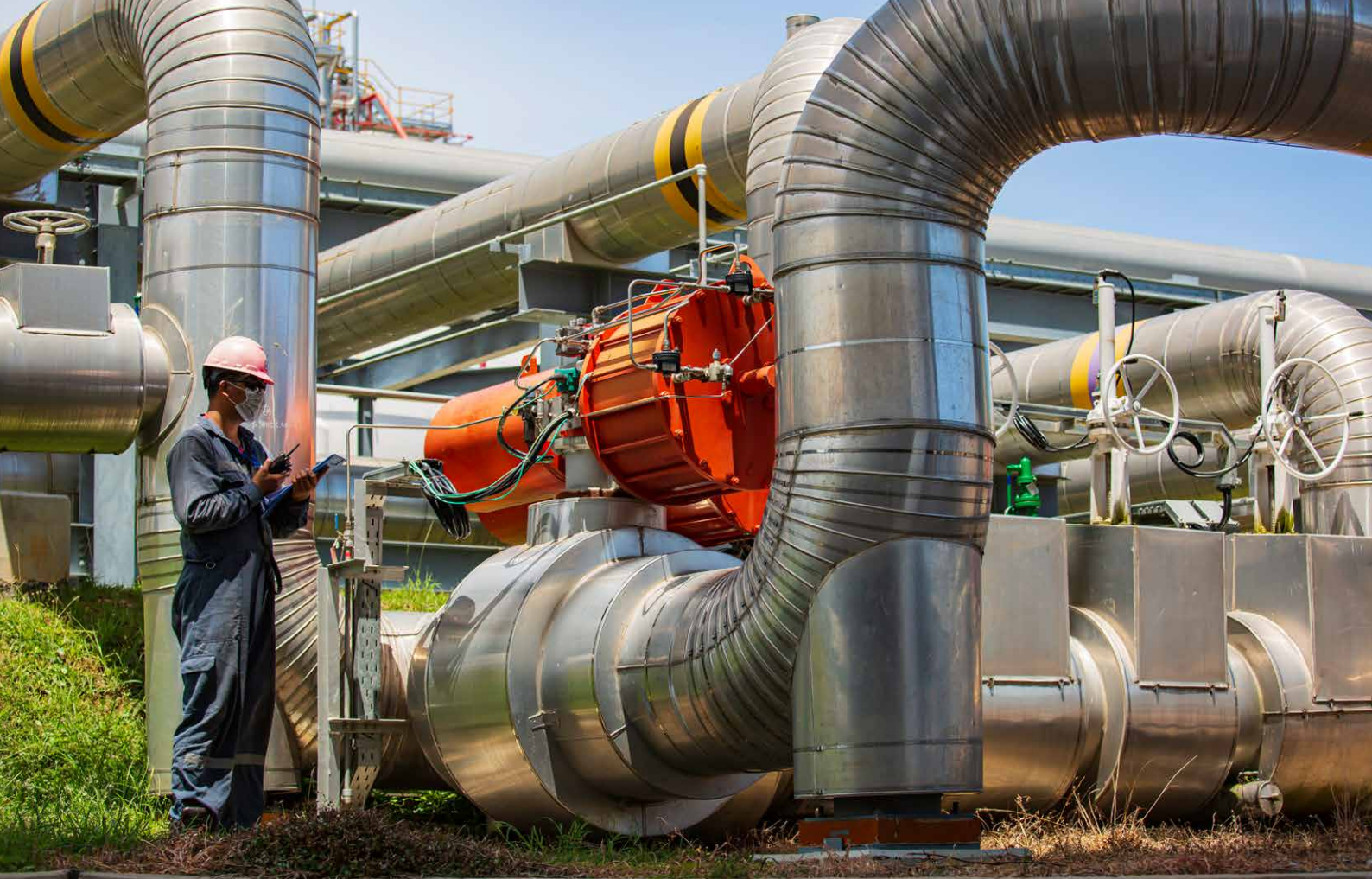
Above: Maintenance on a centrifugal fan.
