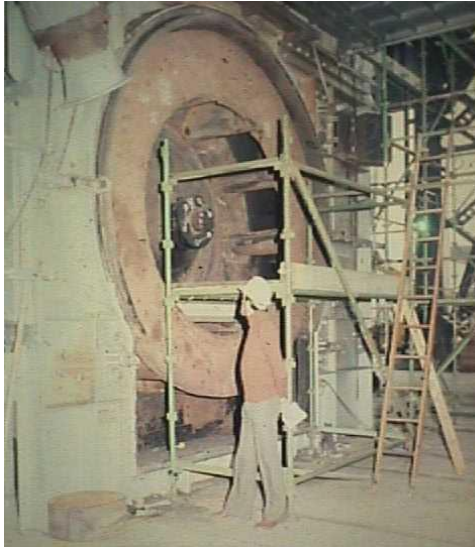
Figure I: fan-type coal mill, showing impeller.
