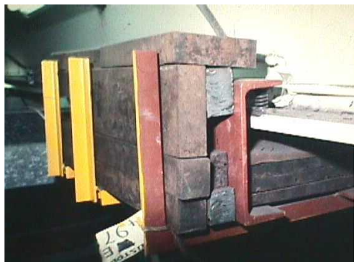
Figure III: typical absorber supported on lower flange of control room beams.
