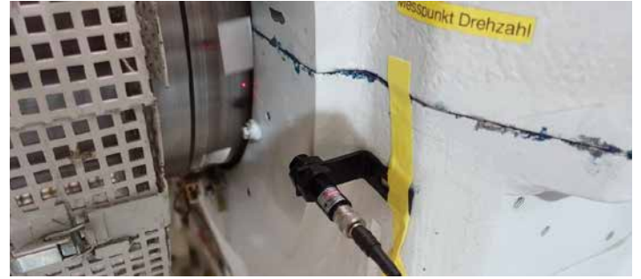
Figure 3: Laser tachometer at the drive end generator bearing.
