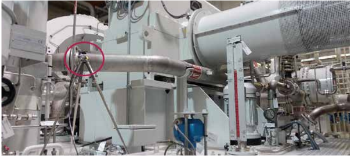
Figure 4: Microphone on the left gear box side looking from the generator towards the turbine.
