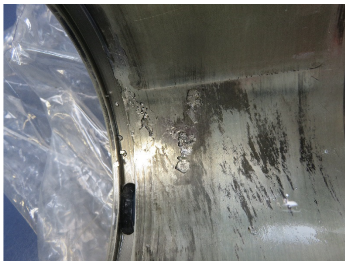
Figure 2. Damaged Coupling End Turbine Bearing.
