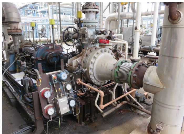
Figure 1. Carbonate Feed Pump G-101-2, Turbine End.
